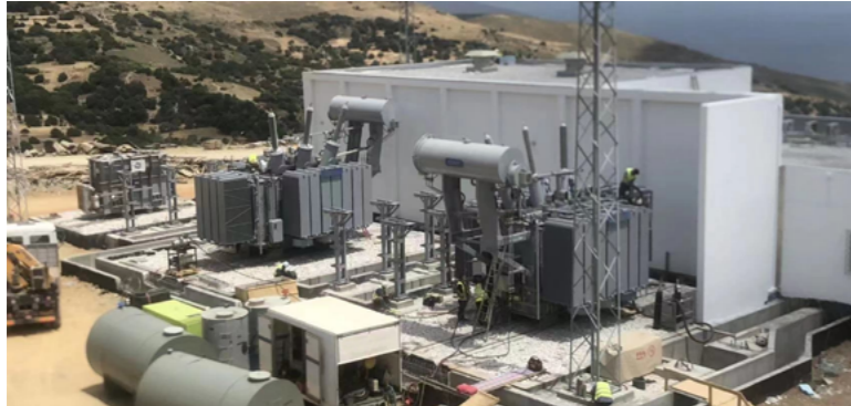
METON New Energy Power Station Transformer project
