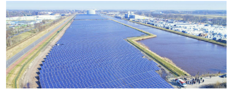
Andijk 15MW Solar Solar Power Plant
