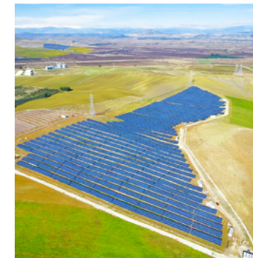
Osmanlye 5.31MW Solar Power Plant
