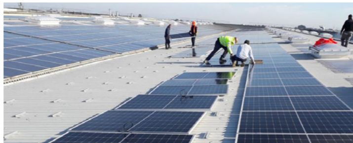
120kW Rooftop Solar Plant
