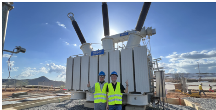
THE PHILIPPINES | Cayanga Bugallon 75MW Solar Power Plant
