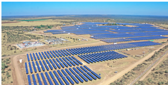
SOUTH AFRICA | Limpopo 64MW Solar Power Station
