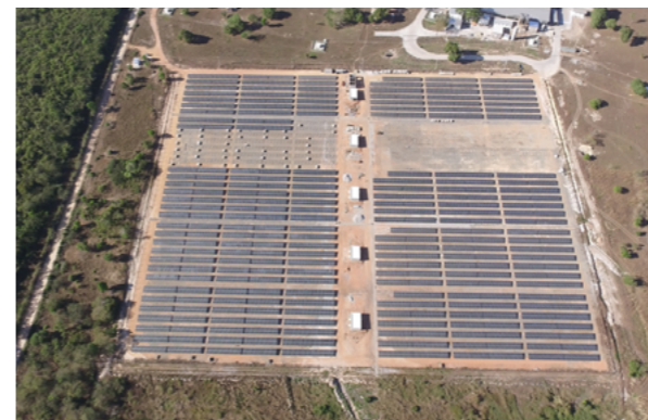
Naturagua 5MW Ground PV Plant
