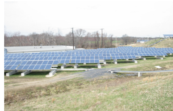
New Jersey Clean Harbors 1.5MW Solar Power Plant
