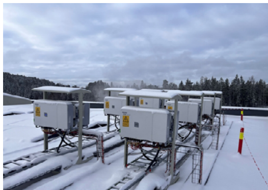
2MW Rooftop Project
