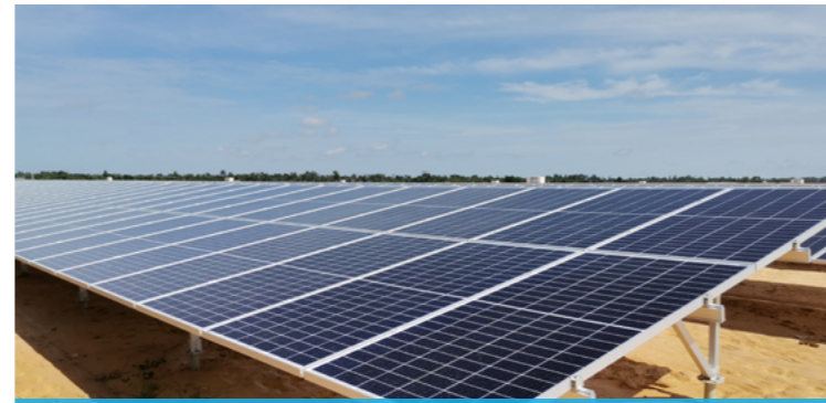
CAMBODIA | Pursat 30MW Ground PV Plant
