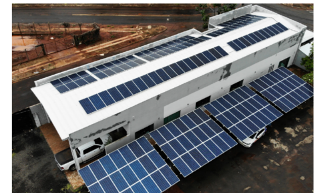
Imbauba 420kW Solar Power Station
