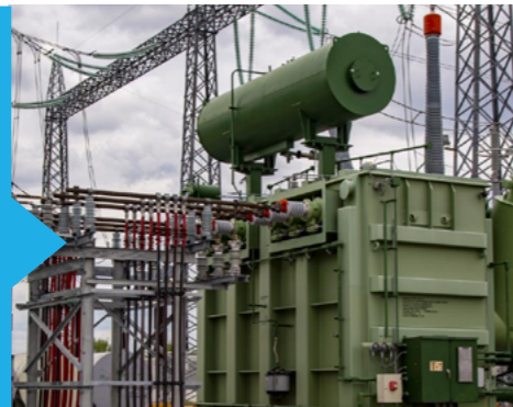
Reynosa wind power station 400kV 225MVA Power Transformer Project
