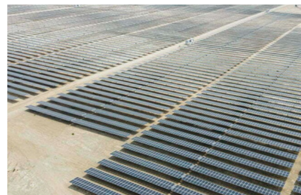
ADANI PHUOC MINH 50MW Solar Power Plant
