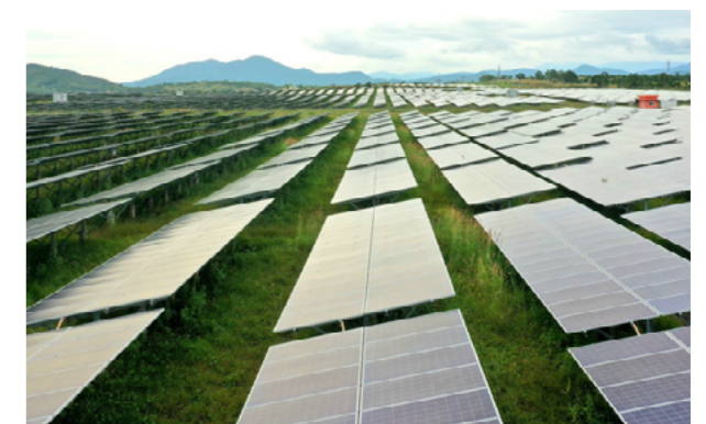
PHAN LAM 36.72MW Solar Power Plant
