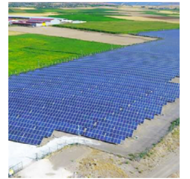
Nevsehir 3.55MW Solar Power Plant
