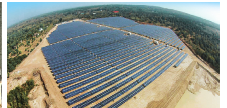
THAILAND | EPD 16MW Solar Power Plant
