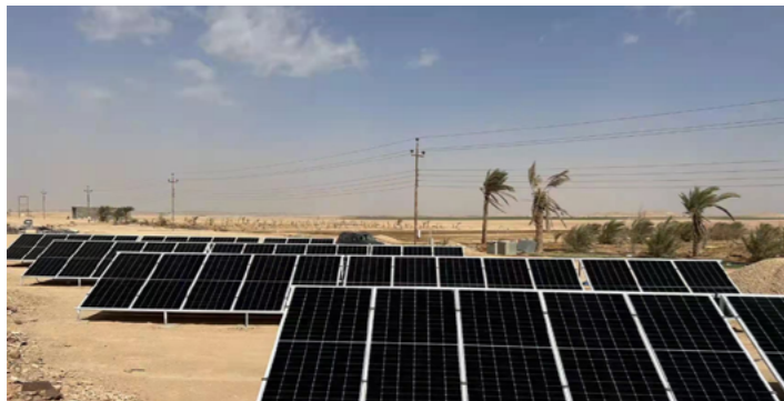
IRAQ | 350kW Off-grid Solar Pumping Project
