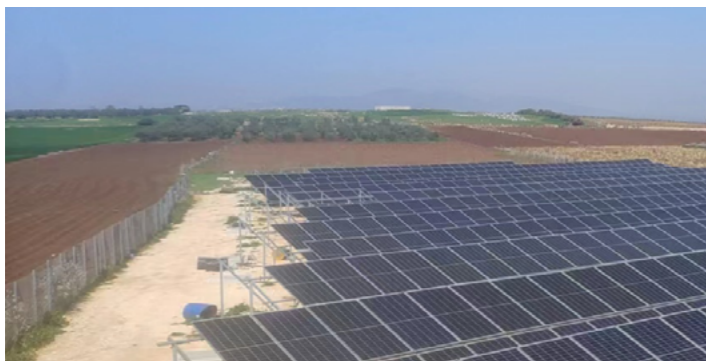
PALESTINE | West Bank 7MW Ground Solar Project
