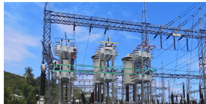
THE PHILIPPINES | NGCP Compostela (CEBU) Substation
