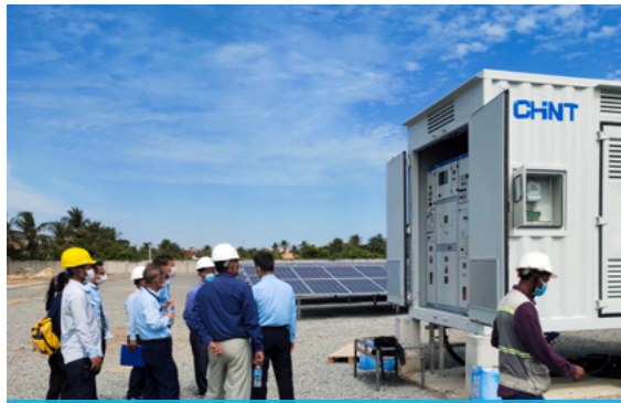
CAMBODIA | 1.8MW Ground PV EPC Project
