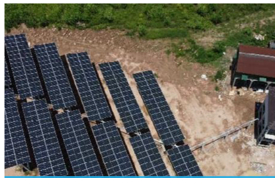
CAMBODIA | Off-grid Village-level Solar Power Project
