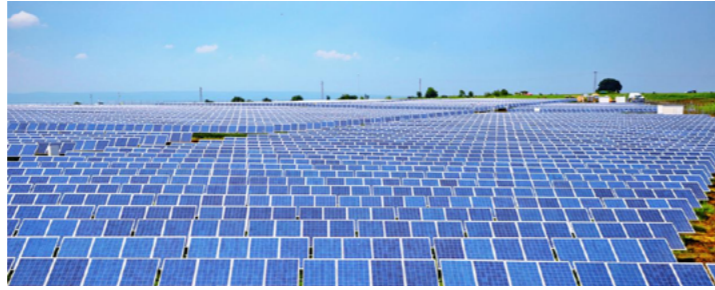
Chargan 3MW Solar Power Plant
