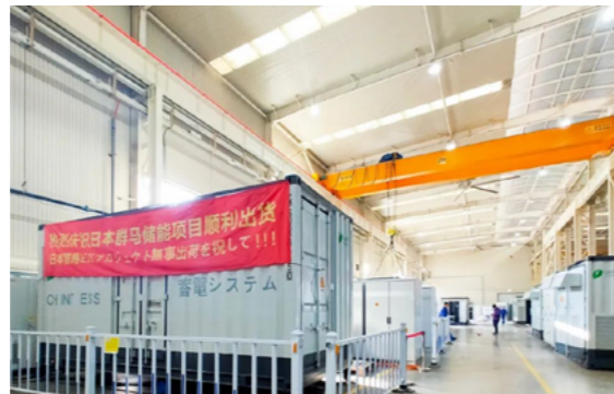
JAPAN | 500kW/2MWh BESS Project
