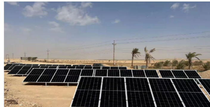
IRAQ | 350kW Solar Sand + PV Pumping Project
