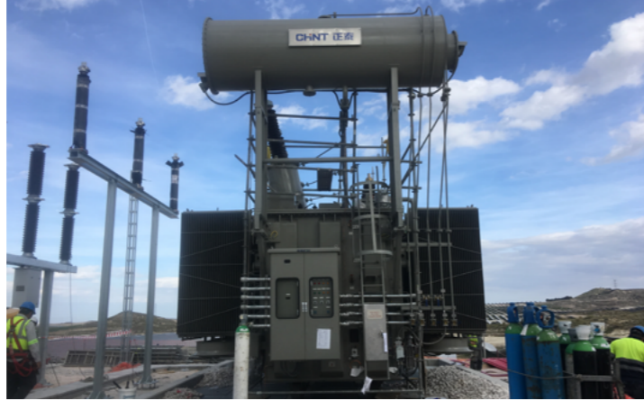
Maetel 5.6MW Solar Power Plant
