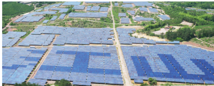
Jiangshan 200MW Forest-Solar Complementary Power Station
