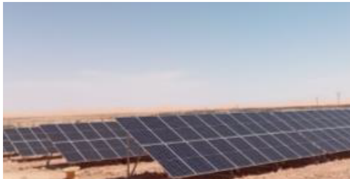
ALGERIA | SONELGAZ 23MW Ground PV Project
