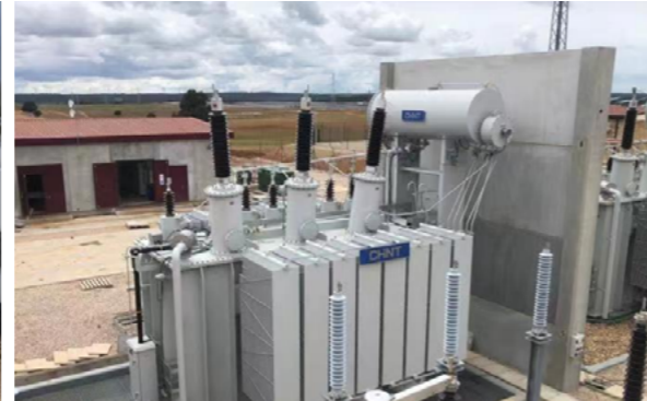
Terna Wind Farm 150kV Power Transformer Project
