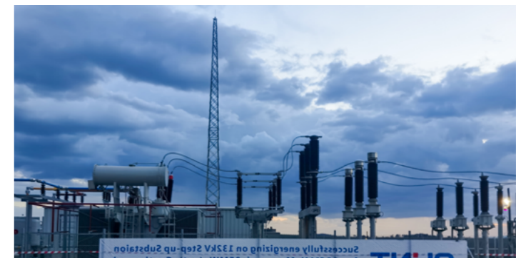
KENYA | KETRACO Sosian Geothermal Power Station Step-up Substation EPC Project
