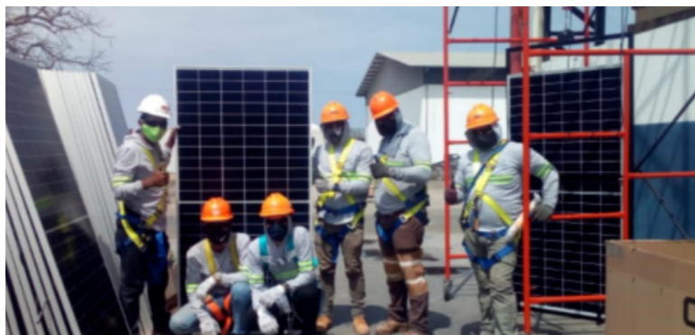
ECOTEC University Rooftop PV Plant
