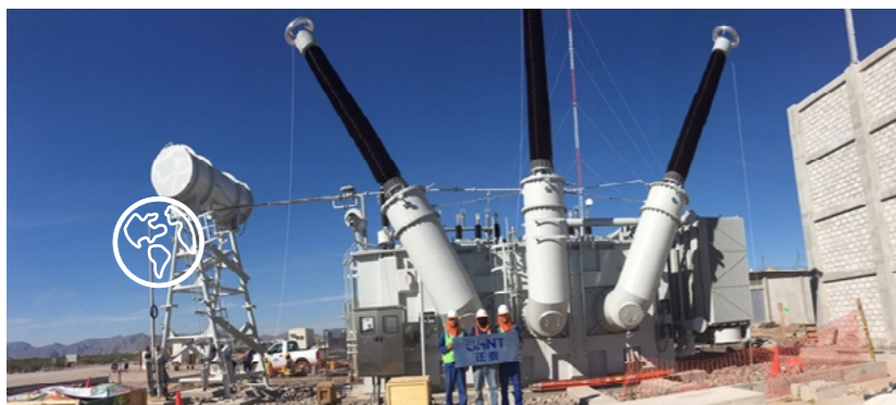
Villanueva III Solar Power Plant
