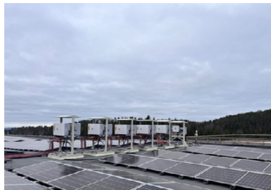
1.1MW Rooftop Project
