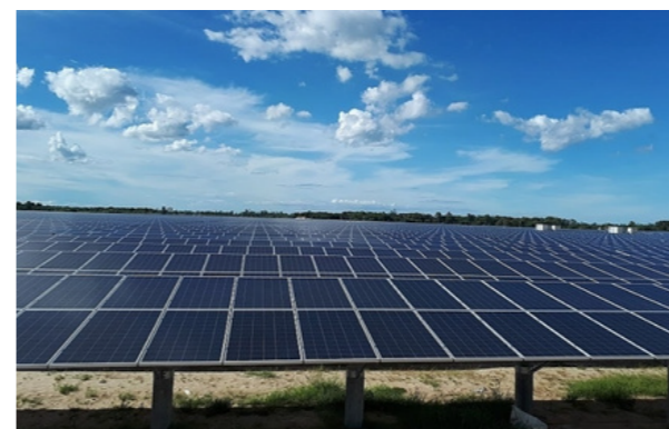
SE SAN 49MW Solar Power Plant
