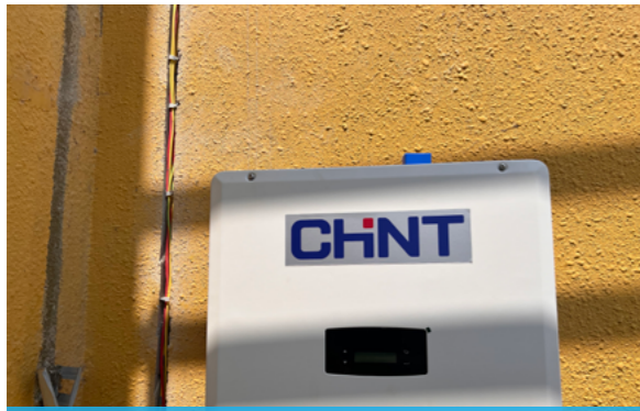
Baku Masazir 20kW Rooftop Project
