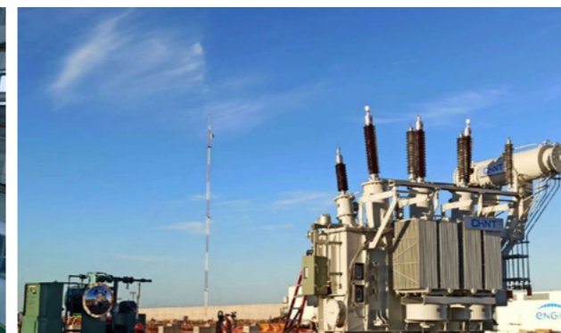
ENGIE 27MW Solar Station Power Transformer Project
