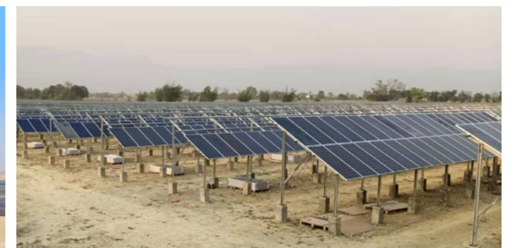
NEPAL | 2.2MW Ground PV Plant
