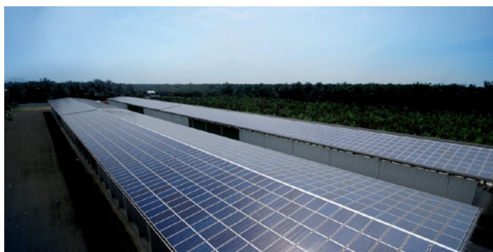
MALAYSIA | K-STRUCTURES Rooftop Solar Power Station
