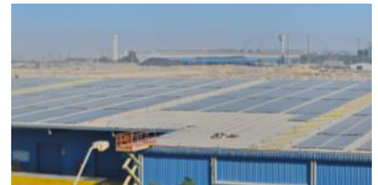
EGYPT | Jushi Fiberglass Manufacture Base 6.9MW Rooftop PV Project
