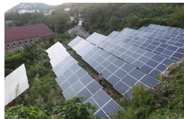
Nanji Island Off-grid Solar Power Station
